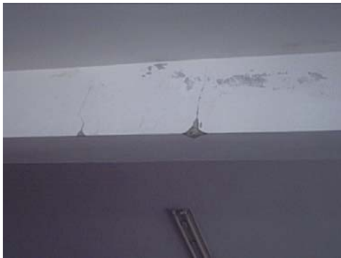
Fig. 4.14: Vertical Cracks in Drop Beams.
