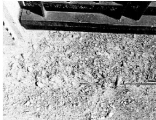
Very Severe Scaling
