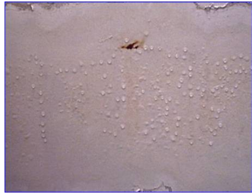
Fig. 4.7: Appearance of Rust on Surface.
