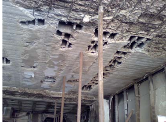
Fig. 3.7: Typical Fire Damages. (IUG Library Building-March, 2008)
