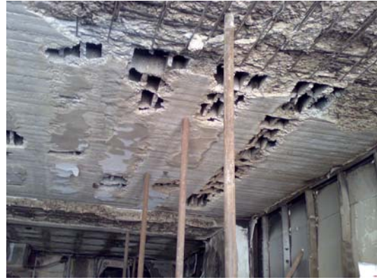
Fig. 3.7: Typical Fire Damages. (IUG Library Building-March, 2008)
