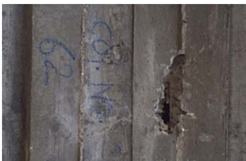
Segregation (Al-Nasser Hospital-Gaza)
