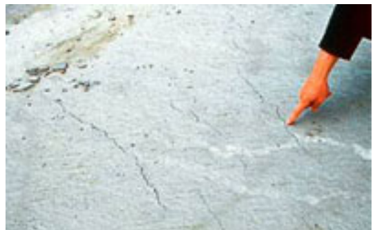
Fig. 3.2: Plastic Shrinkage Cracks. ( www.cement.org/tech/faq_cracking.asp )
