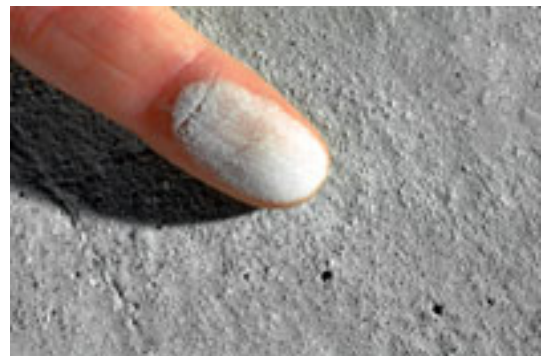
Fig. 3.11: Dusting of Concrete Surface. ( http://www.prairie.com )
