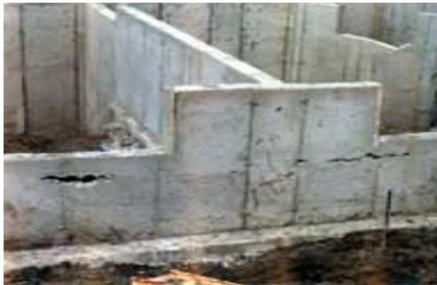
Cold Joints (www.enhance-solutions.com)
