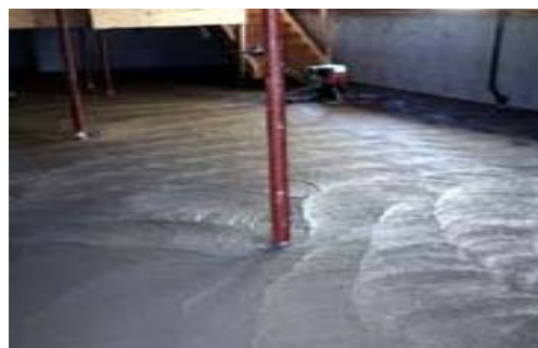
Bad Surface Finish (www.enhance-solutions.com)
