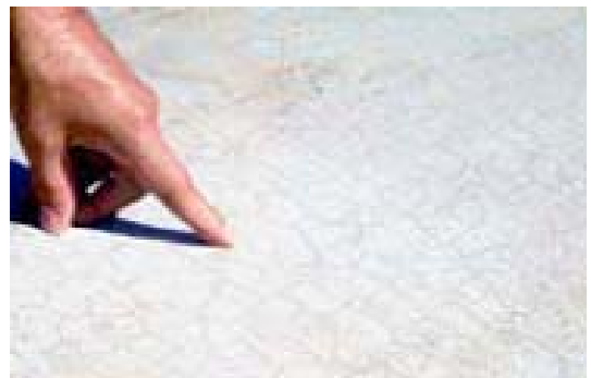
Fig. 3.4: Craze Cracks. (www.prairie.com)
