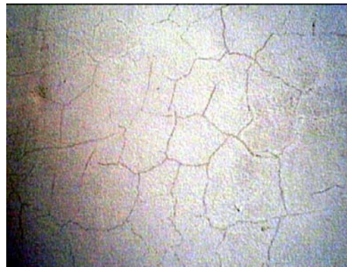
Fig. 4.18: Craze Cracks in External Plaster.
