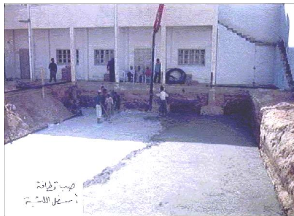
Fig. 4.15: Differential Settlement Cracks at Expansion Joints.
