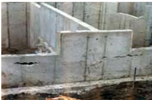
Cold Joints (www.enhance-solutions.com)
