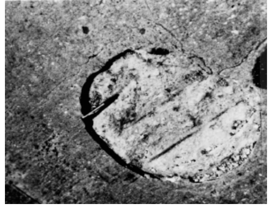
(b) Large Spall
