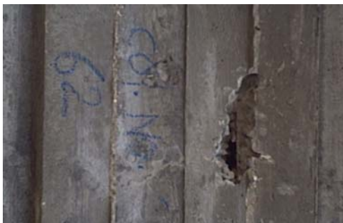
Segregation (Al-Nasser Hospital-Gaza)
