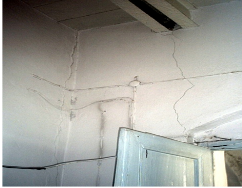
Fig. 4.12: Vertical and Inclined Cracks in Bearing Walls.
