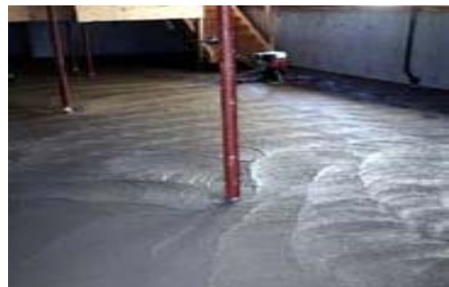
Bad Surface Finish (www.enhance-solutions.com)
