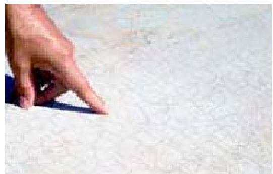
Fig. 3.4: Craze Cracks. (www.prairie.com)
