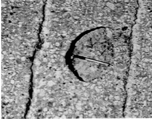
(a) Small Spall
