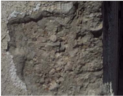
Fig. 4.6: Deterioration of Concrete.
