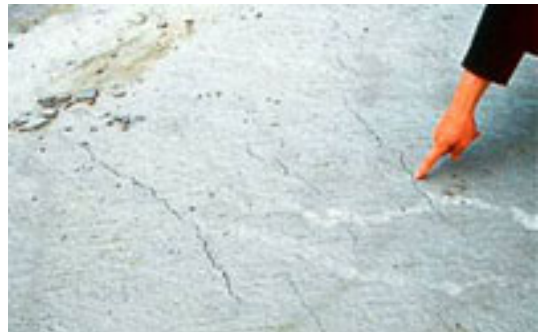
Fig. 3.2: Plastic Shrinkage Cracks. ( www.cement.org/tech/faq_cracking.asp )
