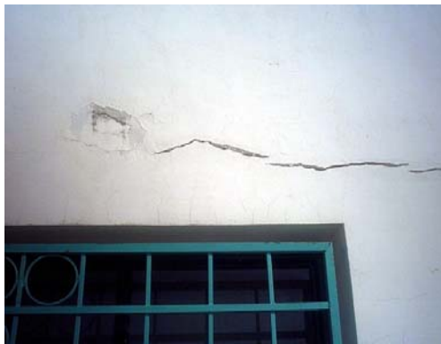
Fig. 4.17: Horizontal Cracks Between Windows Concrete Lintel and Block Works.
