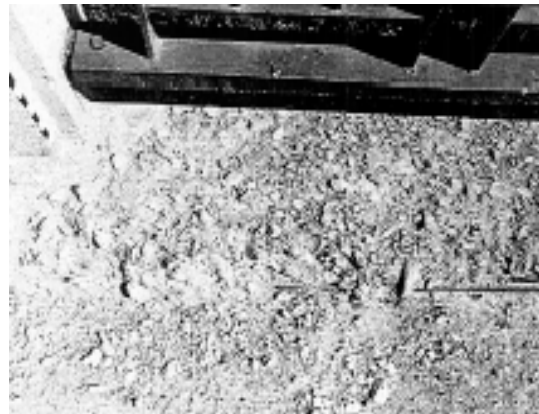
Very Severe Scaling
