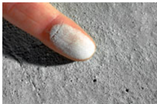
Fig. 3.11: Dusting of Concrete Surface. ( http://www.prairie.com )
